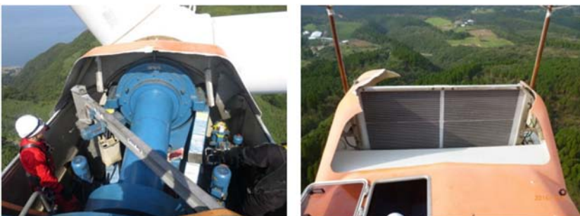
FIGURE 1 Damage to the nacelle cover during the typhoon at Minamiosumi wind farm 12 [Colour figure can be viewed at wileyonlinelibrary.com ]
