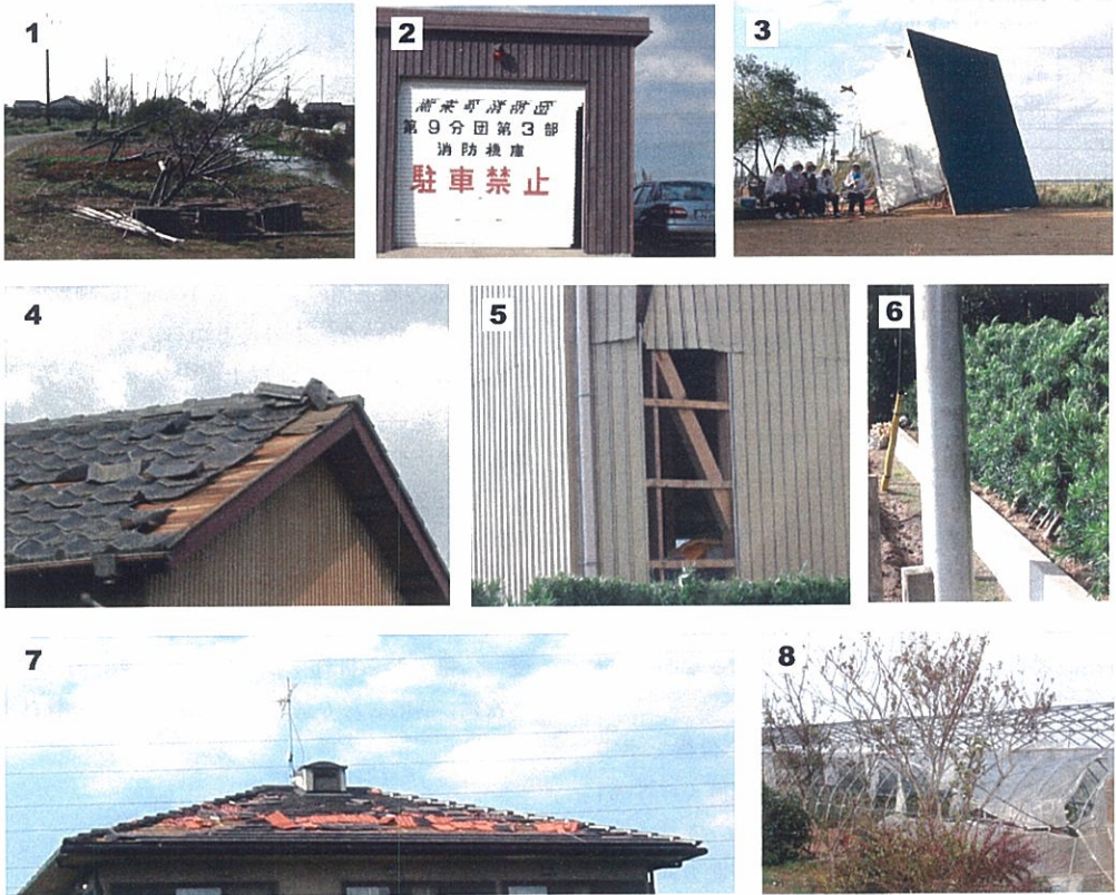
Fig. 5 送電鉄塔の倒壊現場に近い場所での建屋と樹木の被害状況 (Damage of houses and trees near the site of collapsed power transmission towers)
